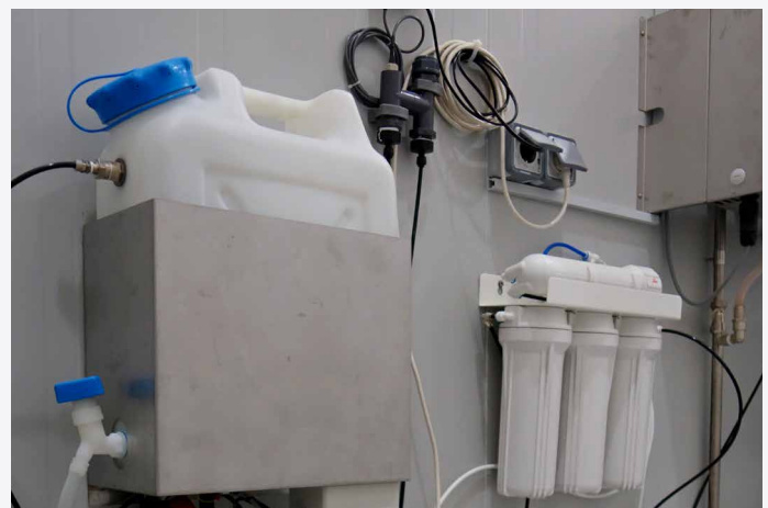
Water Treatment systems
